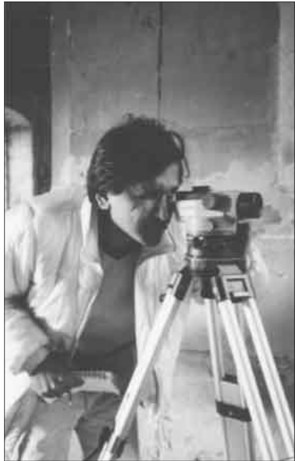
Mohammed Jamal from Chanton Engineering using a theodolite to survey the levels of the upper surfaces of the vaults of Hawksmoor's crypt exposed in the recent excavations of the nave floor.
